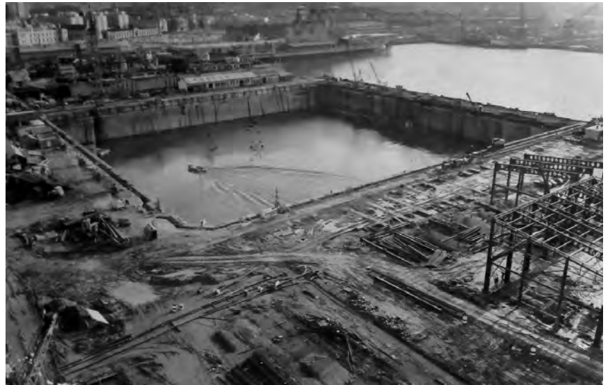
Fig. 150. Cofferdam completed. TNA, CM 20/61 (1973–74). PSA: Devonport: Works Projects. Photograph albums. Nuclear Submarine Refit Complex book no. 1. Submarine Refit Complex December 1974. Reproduced with the permission of The National Archives.
