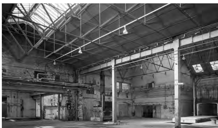
Fig. 69. BB96/03867. Devonport South Yard South Smithery (S126) photograph of interior central building, view from southeast (29 Feb 1996). ©Crown copyright.HE.
