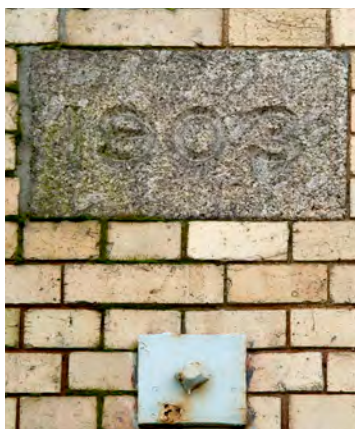
Fig. 183. DP13021. Devonport South Yard: photograph (8 Feb 2011) of Building S173 recorded before demolition. Stone dated 1903 on the west elevation. ©Historic England.
