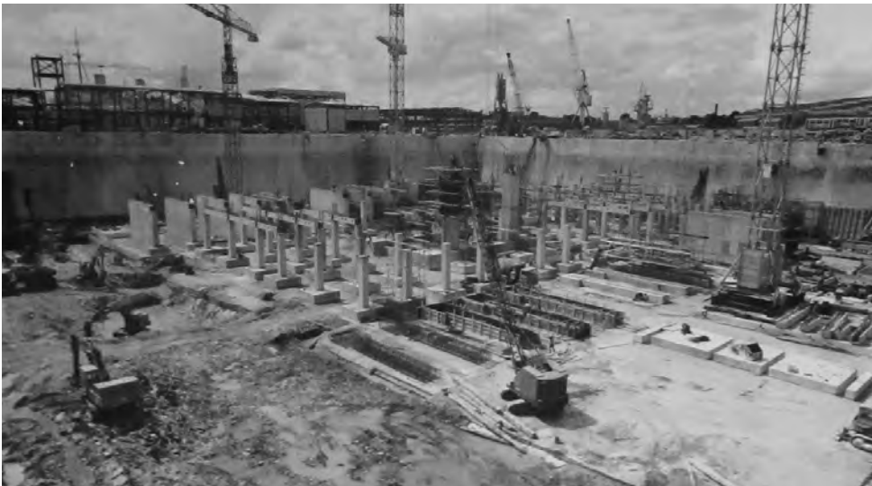
Fig. 151. Submarine Refit Complex (May 1975). TNA, CM 20/62 (1975). PSA: Devonport: Works Projects. Photograph albums. Nuclear Submarine Refit Complex book no. 2. Reproduced with the permission of The National Archives.
