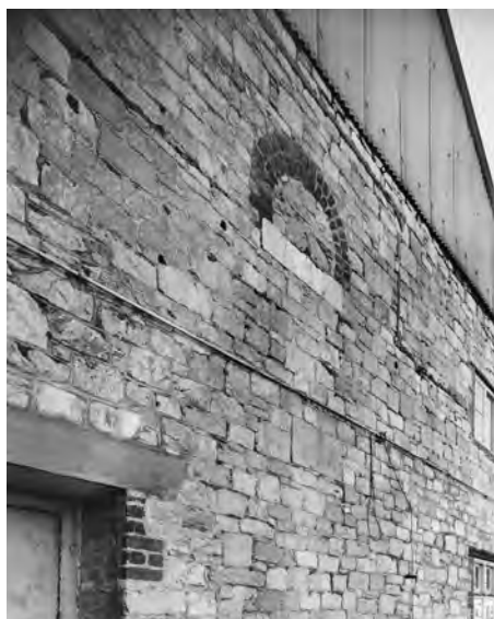
Left: Fig. 68. BB96/03859. Devonport South Yard South Smithery (S126) photograph detail of evidence of the line shaft on the north side of central building (29 Feb 1996). ©Crown copyright.HE.
