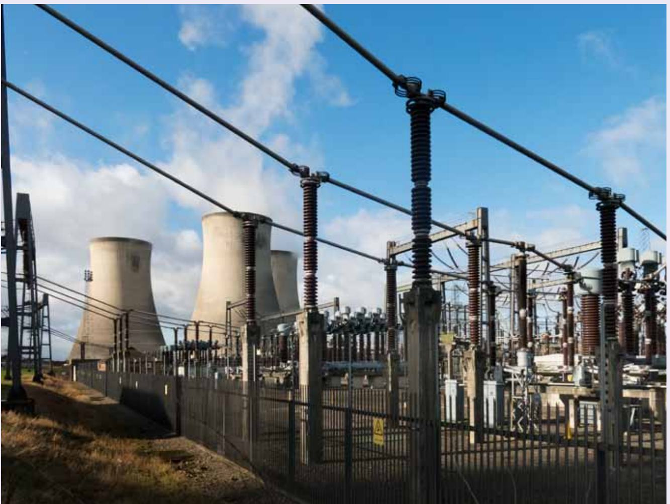
Didcot 'A' Power Station, Didcot, Oxfordshire (5A3). Photo by Steve Cole, © English Heritage.
