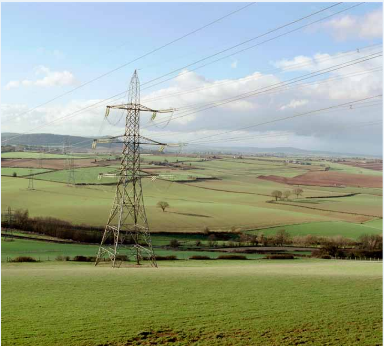
Electricity pylons at Aston Ingham, Herefordshire. Photo by Peter Williams, © English Heritage
