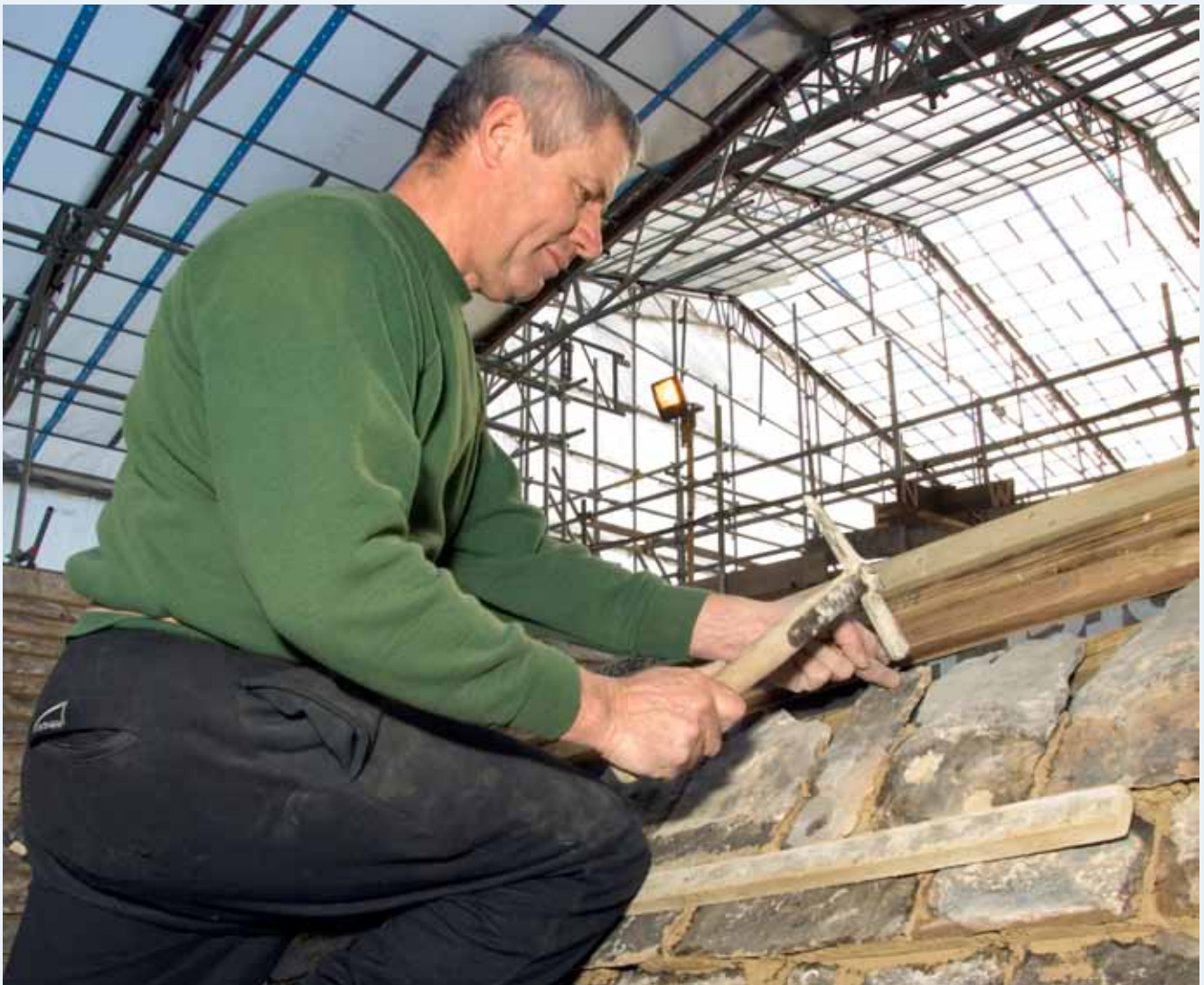
Collyweston slate being installed at Apethorpe Hall, Northamptonshire. Photo by Patricia Payne, © English Heritage.
