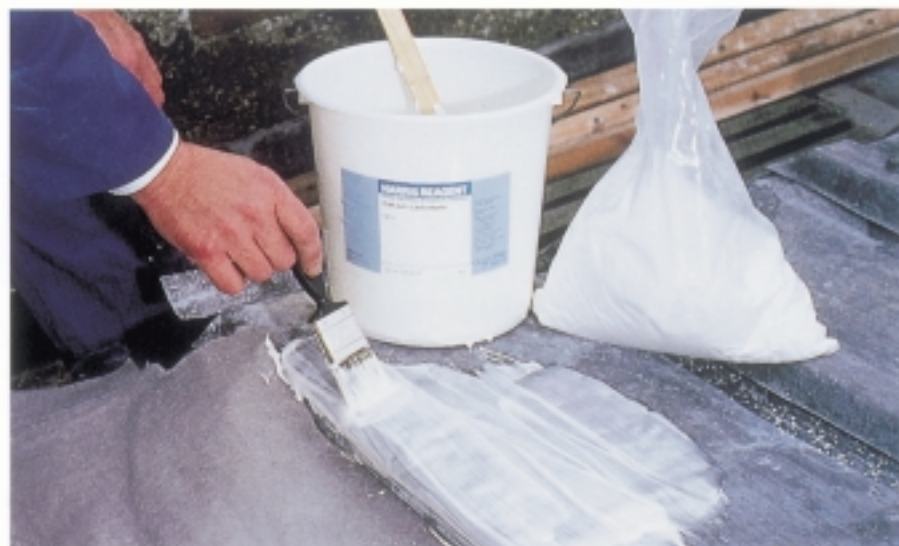
Figure 30 Applying the chalk slurry to the fresh lead. The coating thickness is sufficient when the surface of the lead can no longer be seen.
