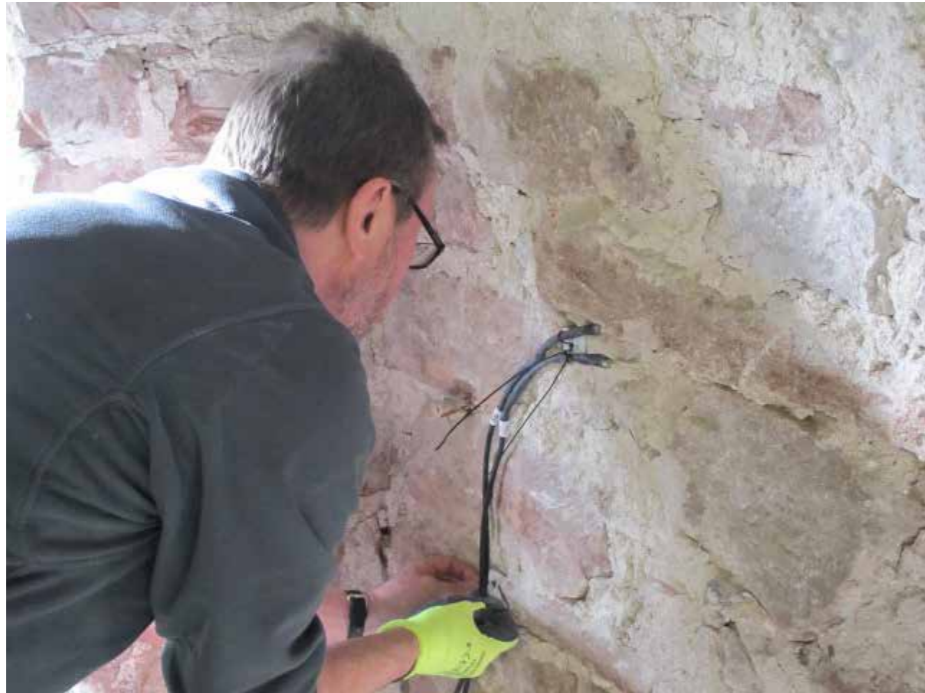
Right: Fixing the sensors at Chapel Street, Appleby, prior to the installation of lime hemp insulation. © Historic England
