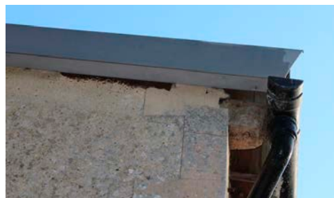
Figure 11: End of fascia with acute corner and incomplete closure
