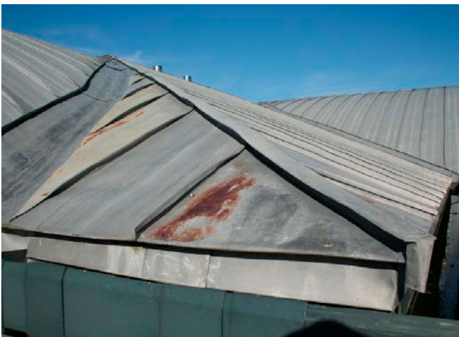
Figure 12: Discolouration of lead-rich terne-coated stainless steel
