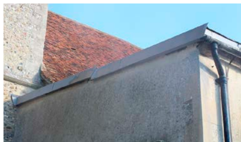
Figure 10: Straight verge fascia contrasts with uneven masonry
