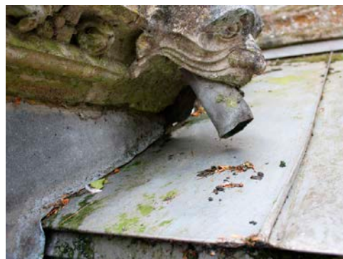
Figure 3: Awkward detail at verge with water running into upstand
