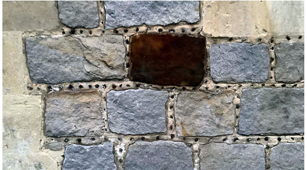
Figure 52: Church of St Michael and All Angels, Pirbright. Sarsen stone and ironstone with ironstone galleting.
