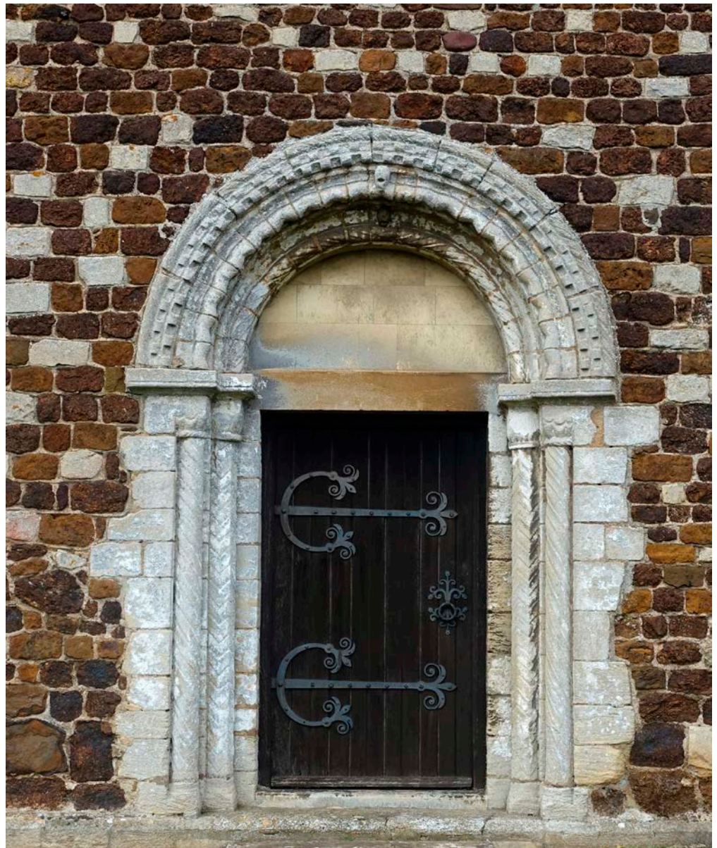
Figure 41: Church of St Mary, Wimbotsham. Totternhoe Stone doorway. Carstone with Chalk Block wall.
