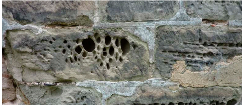
Figure 27: Weathering and exfoliation damage to sandstone.
