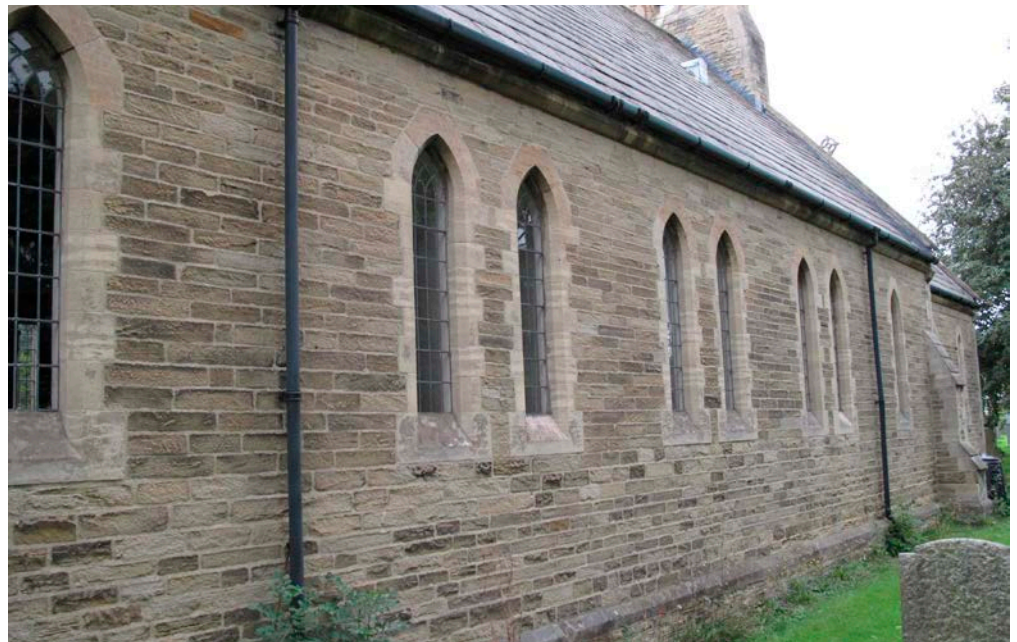
Figure 15: Church of St John the Baptist, Stamford Bridge. Pennine Coal Measures Sandstone.
