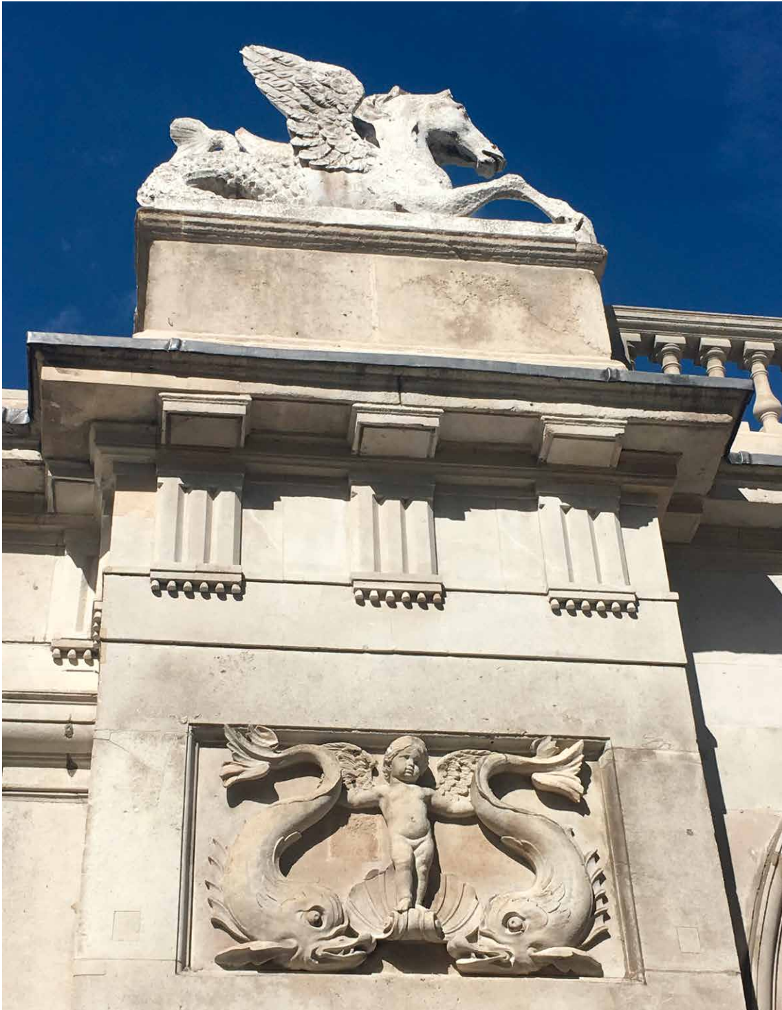
Old Admiralty Buildings, Greater London. The sea-horses or hippocampi on the Adam Screen (1760) have been cleaned and repaired. © Carlile Associates
