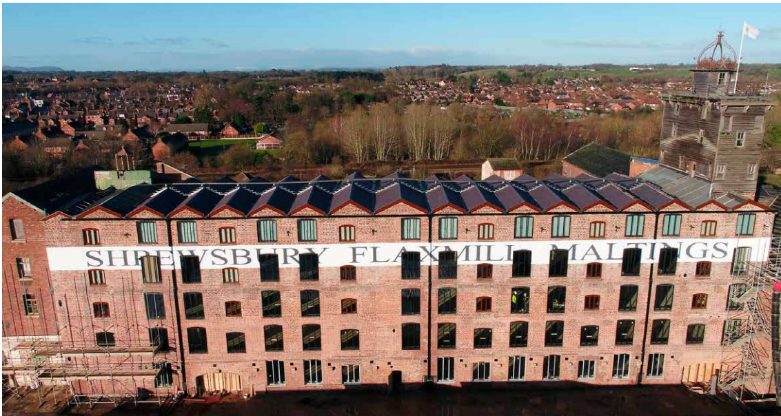
Shrewsbury Flaxmill Maltings, Shropshire. Historic England has repaired the Main Mill to create 28,000 square feet of commercial space. © Historic England Archive
