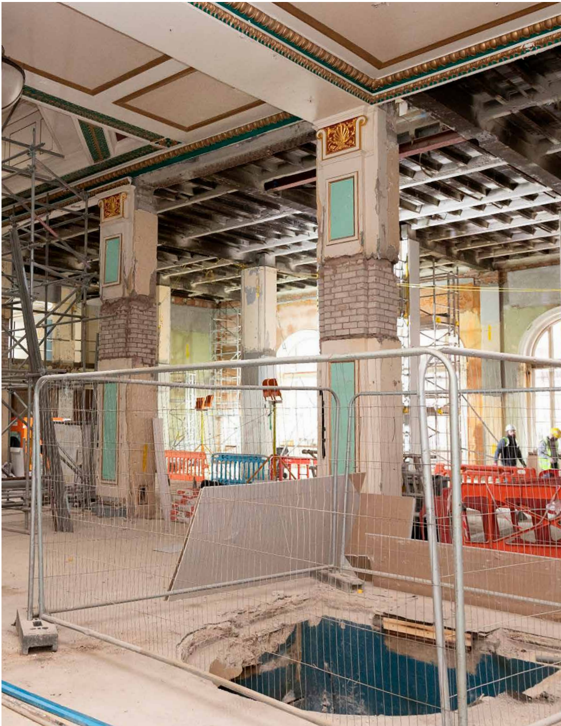
India Buildings, Liverpool (Grade II*). The interior being converted into a Government Hub for HMRC and other bodies. © HMRC
