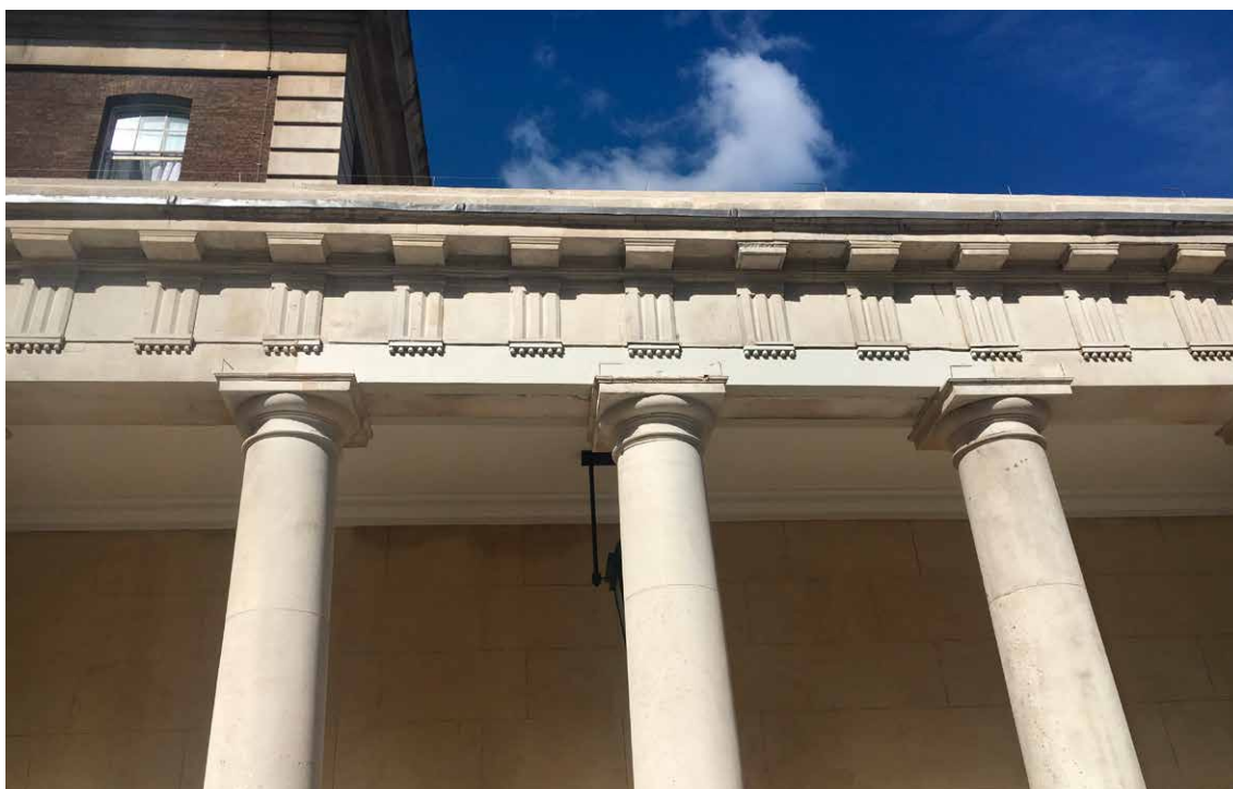
Old Admiralty Buildings, Greater London. Repair work on the Adam Screen, now part of the Cabinet Office. © Carlile Associates
