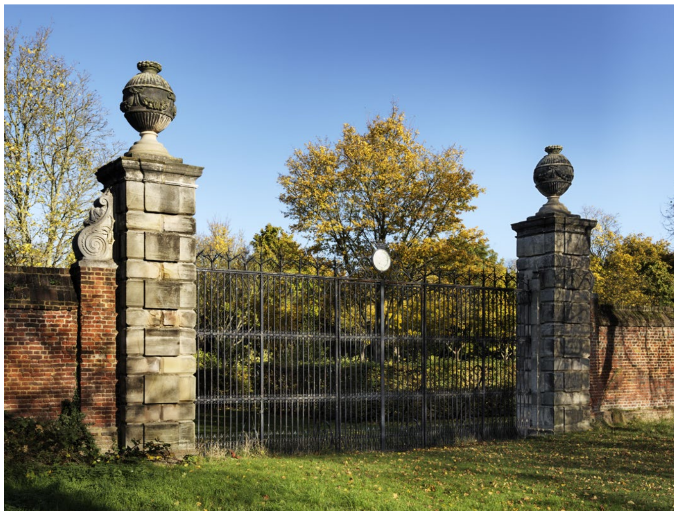
The wrought iron gates at Ham House are heavily corroded and have lost elements of their decorative ironwork. The decorative finish is heavily degraded and in need of renewal to protect the remaining fabric.
