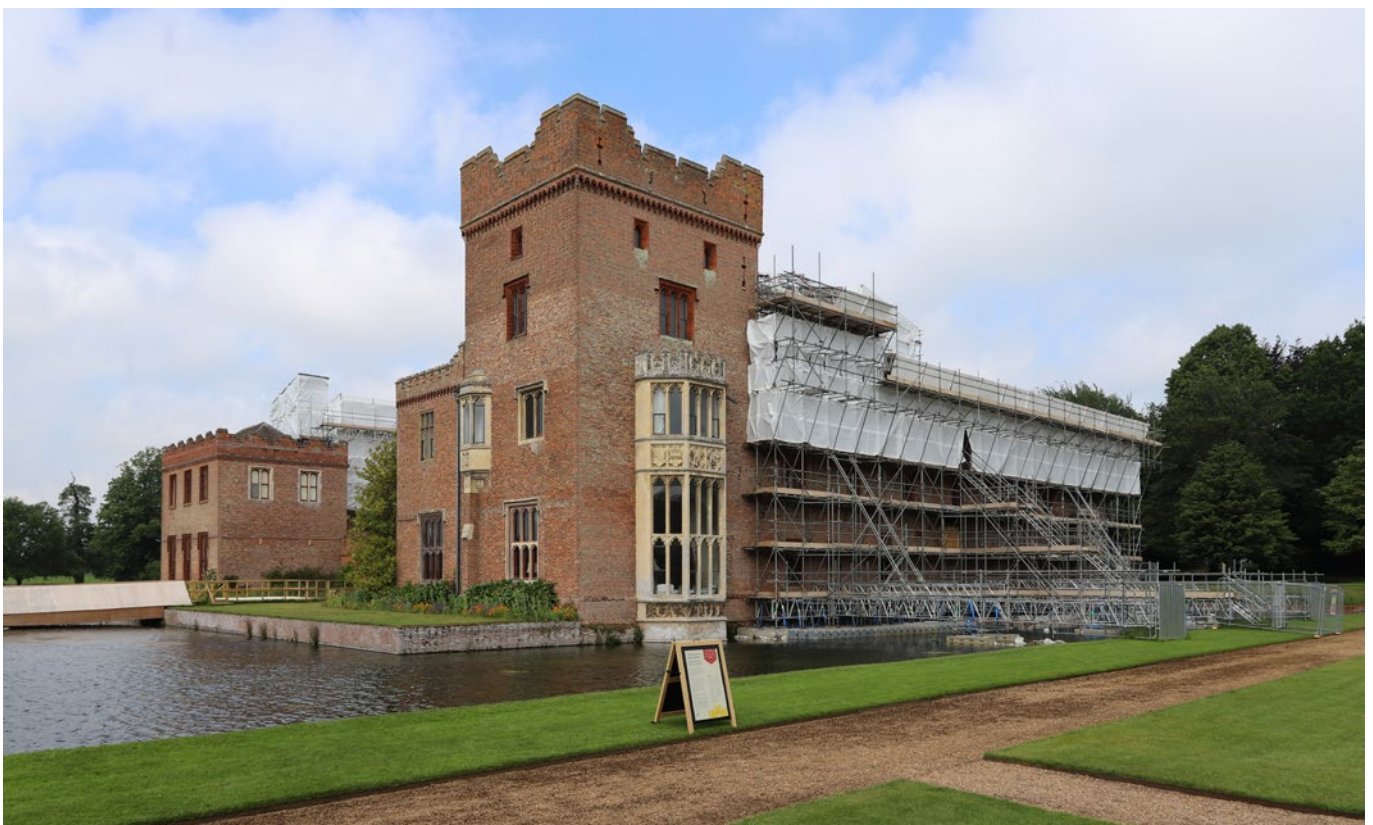
Scaffolding surrounds the hall during the roof restoration project at Oxburgh Hall, Norfolk. © National Trust Images/Mike Selby
