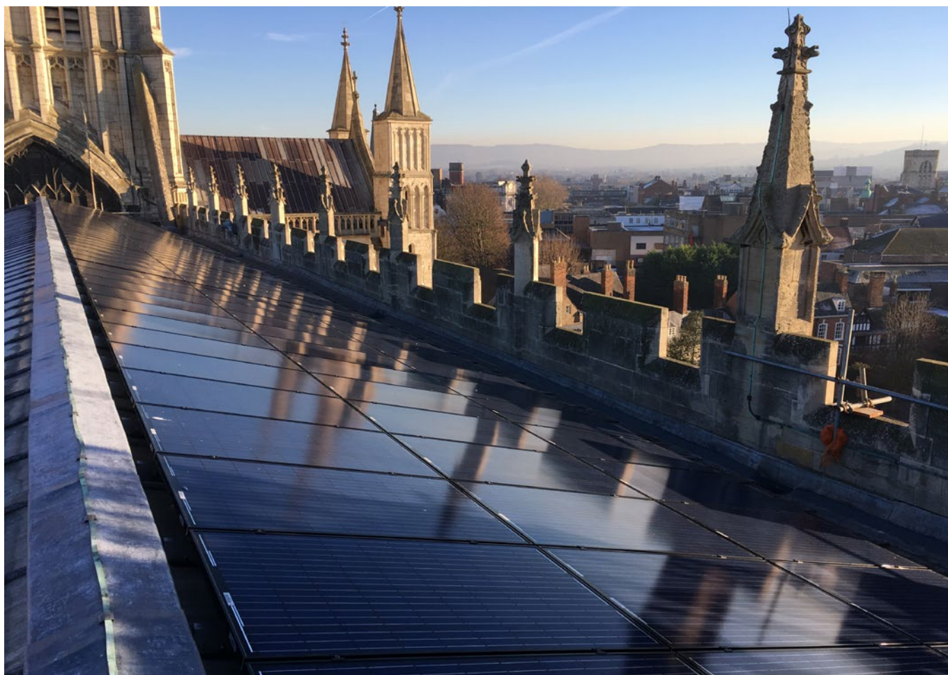
Photovoltaic panels on the south-facing slope of Gloucester Cathedral's medieval roof. © St Ann's Gate Architects
