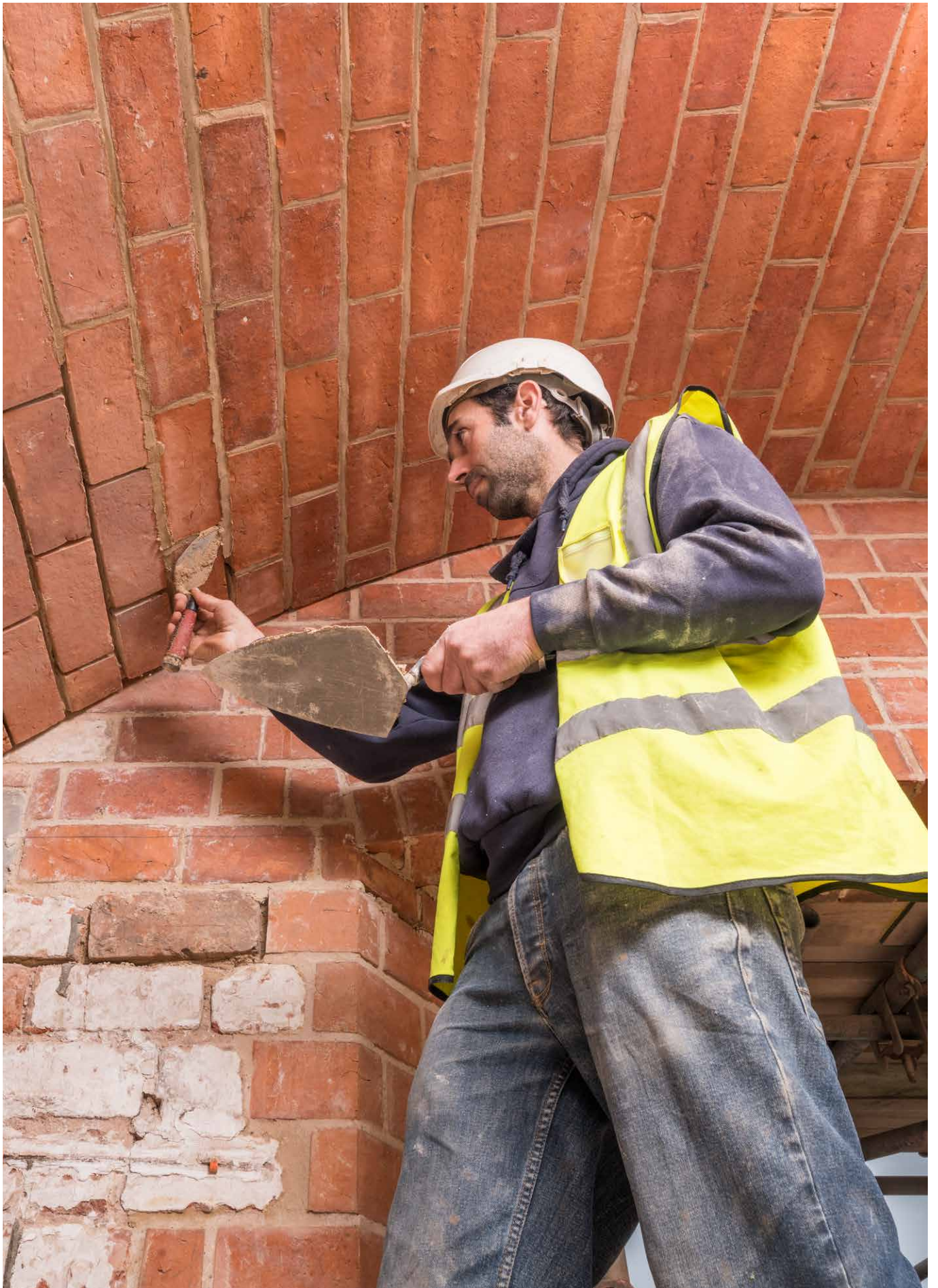
Shrewsbury Flaxmill Maltings, Ditherington, Shropshire. Rebuilding and repointing a brick vaulted arch.
