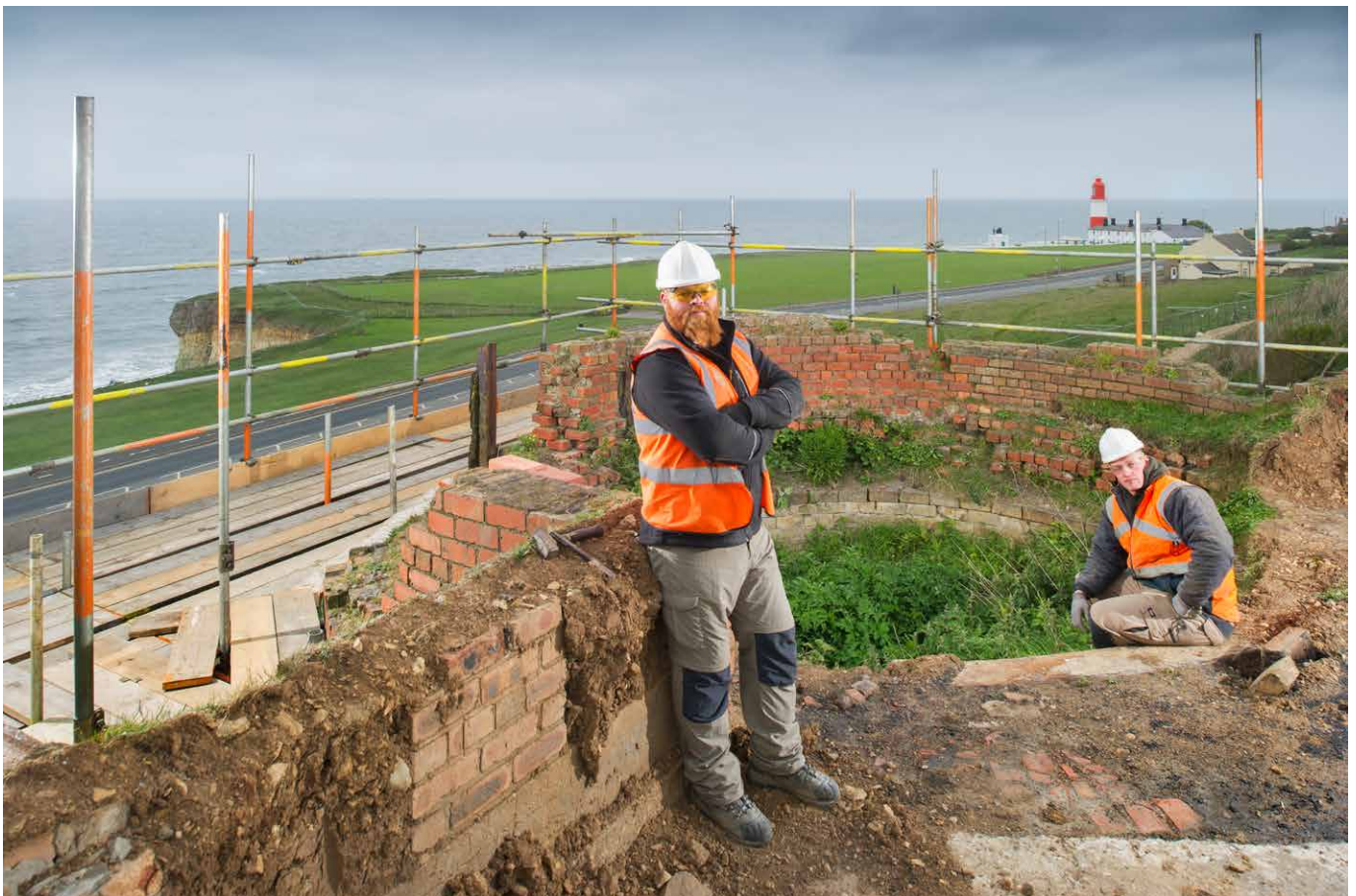
Conservation work being undertaken at Marsden Lime Kilns, Marsden, South Tyneside. © Historic England
