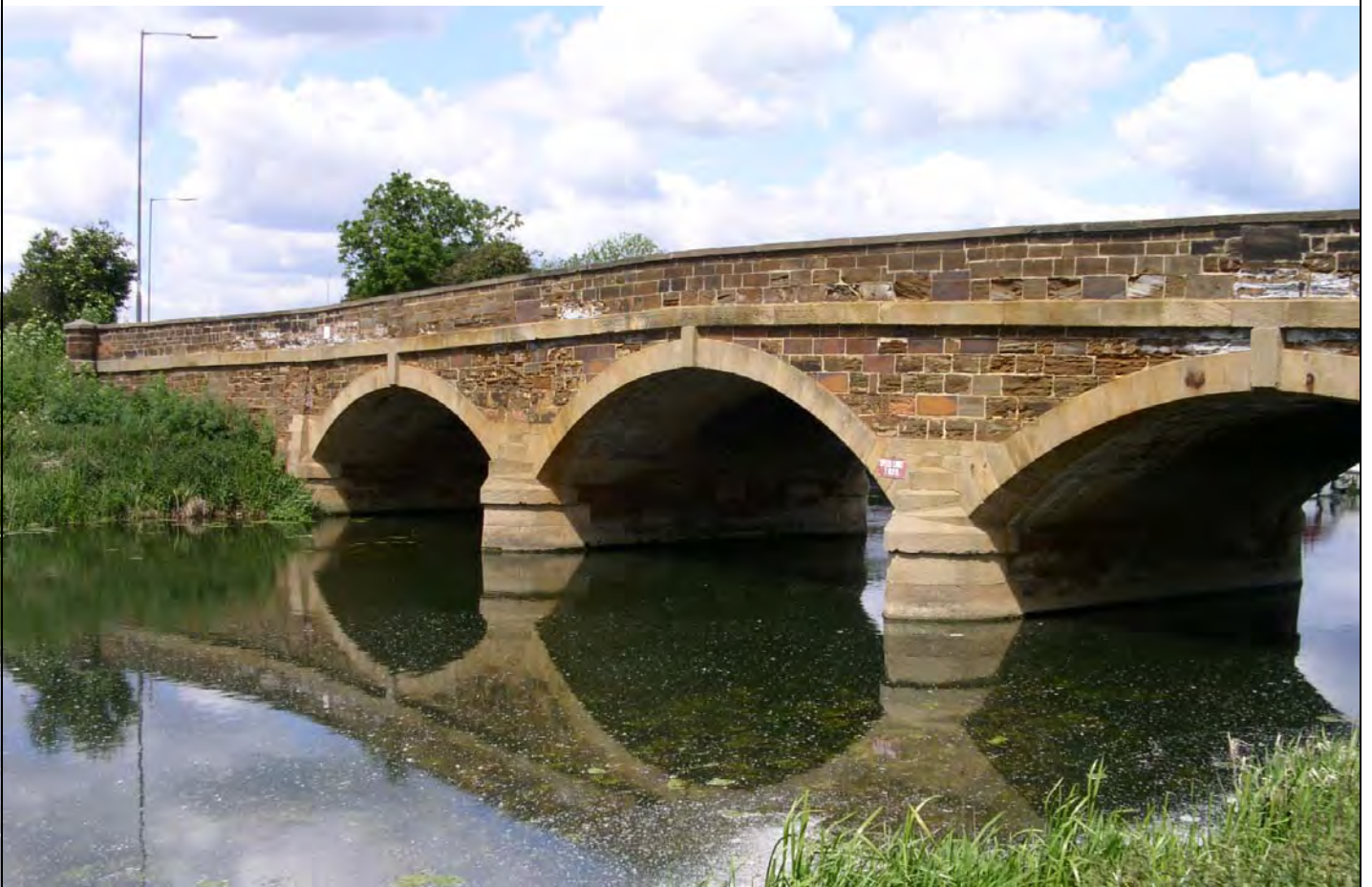
A1 Tempsford Bridge, River Great Ouse, Bedfordshire, Scheduled Monument and Trunk Road
